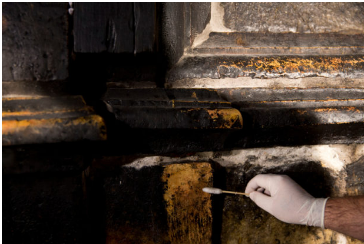
A Greek expert works in renovation of Jesus' tomb in the Church of the Holy Sepulchre in Jerusalem's old city, Monday, June 6, 2016. A team of experts has begun a historic renovation at the spot where Christians believe Jesus was buried, overcoming longstanding religious rivalries to carry out the first repairs at the site in over 200 years. The project, which began Monday, will focus on repairing, reinforcing and preserving the Edicule — the ancient chamber housing Jesus' tomb in Jerusalem's Church of the Holy Sepulchre. It is the first such work at the tomb since 1810, when the shrine was restored and given its current shape following a fire. (AP Photo/Ariel Schalit)
